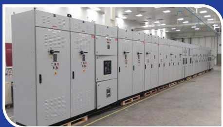
PCC Panel / Switchgear Panel
