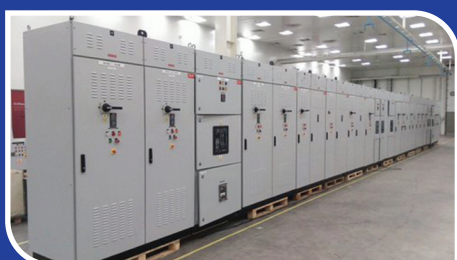
PCC Panel / Switchgear Panel
