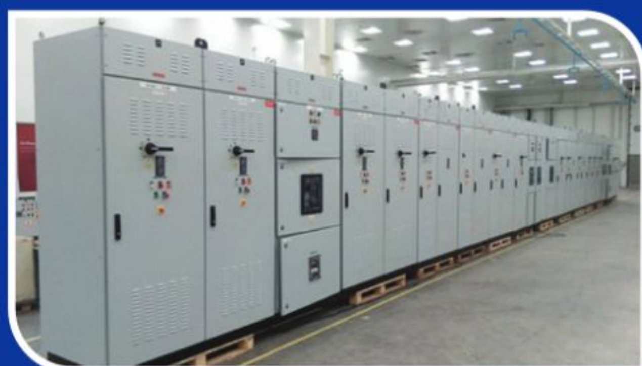
PCC Panel / Switchgear Panel
